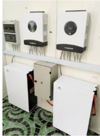
12KW System in Nigeria 🇳🇮
