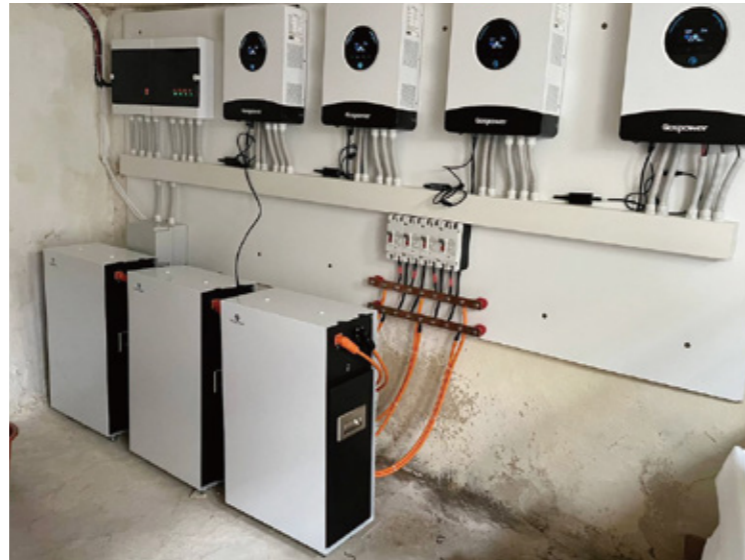
24KW System in Philippines 🇵🇭
