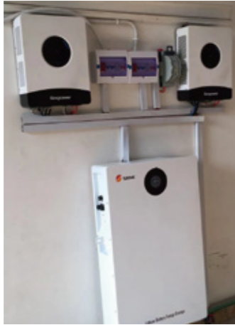
12KW System in Lebanon 🇱🇧
