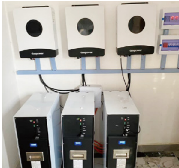
18KW System in Lebanon 🇱🇧
